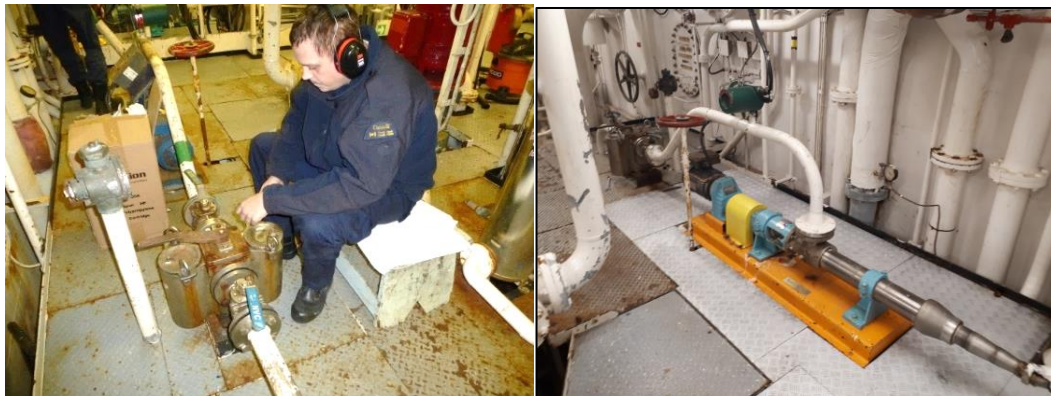
Figure A4. Seawater passes through a filter (in front of engineer) before going to the pump (on orange platform). When the ship is in sea-ice the flow is switched from one filter to the other to allow the necessary frequent clearing out of slush from the filter. Photos are from previous years, but is the same strainer configuration for 2023.
