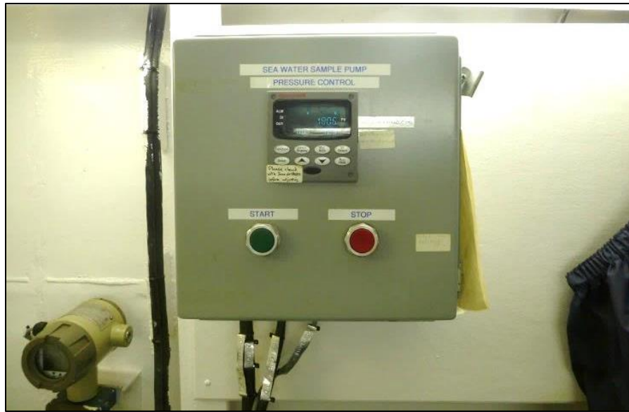
Figure A3. Honeywell controller for the pump, located in the TSG lab.
