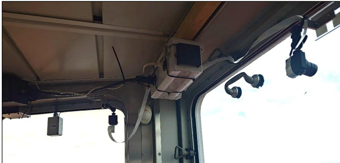
Figure 3.9.3-1: Location of SSICR with forward and side looking lenses on the starboard side of the bridge.
