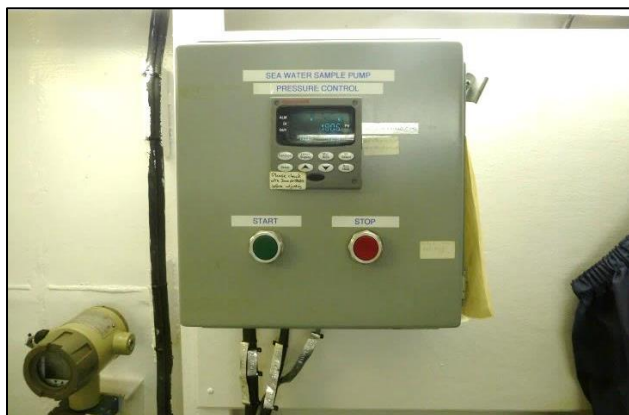
Figure 4.4.1-5. Honeywell controller for the pump, located in the TSG lab.
