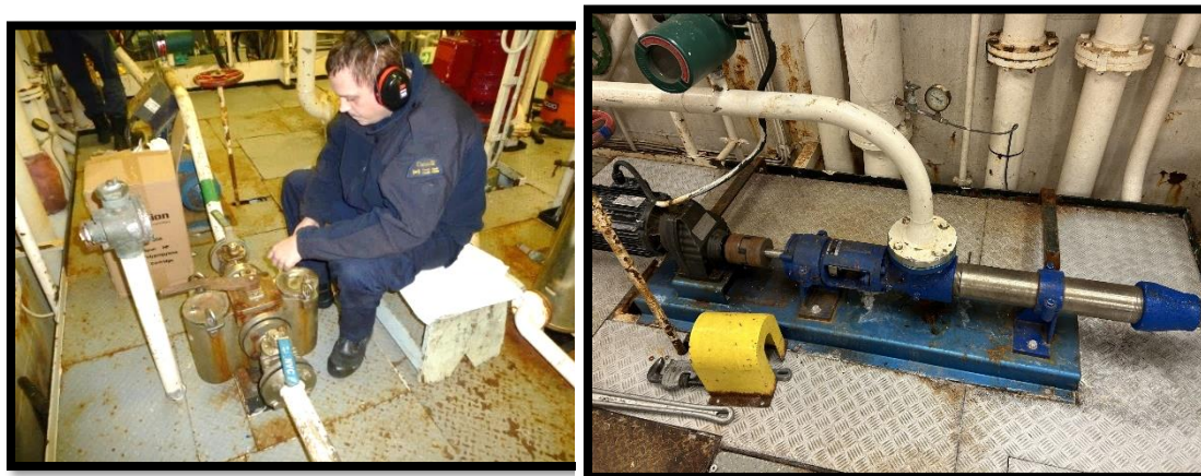
Figure 4.4.1-2. Seawater passes through a filter (in front of engineer) before going to the pump (on blue platform). When the ship is in sea-ice the flow is switched from one filter to the other to allow the necessary frequent clearing out of slush from the filter. Photos on left from previous years, the photo on right from 2025
